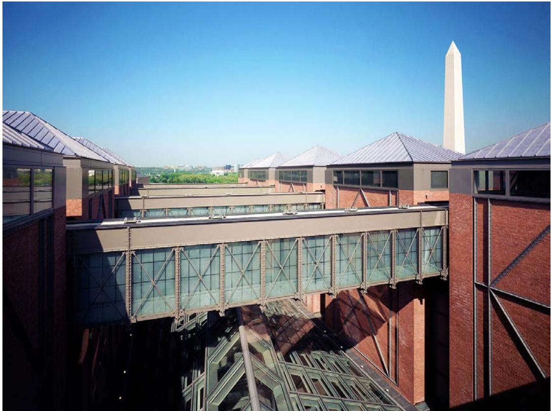
Traditional ground-supported scaffolding wasn't an option due to the glass atrium below the bridges.
