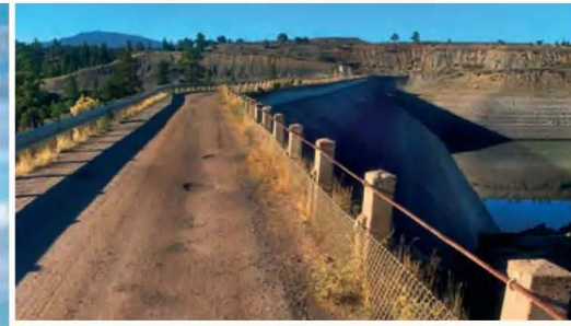
The narrow access road at the top of the dam where the platforms were deployed from and the rigging set up.
